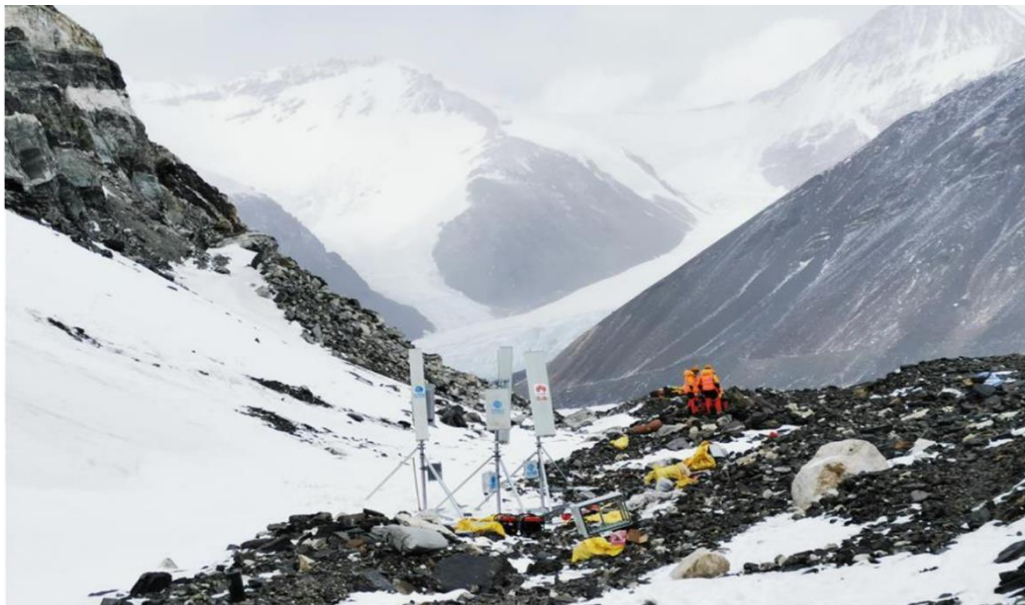
Figure 22 The 5G base station near the Advance Base Camp on Mount Qomolangma at an altitude of 6,500 meters
